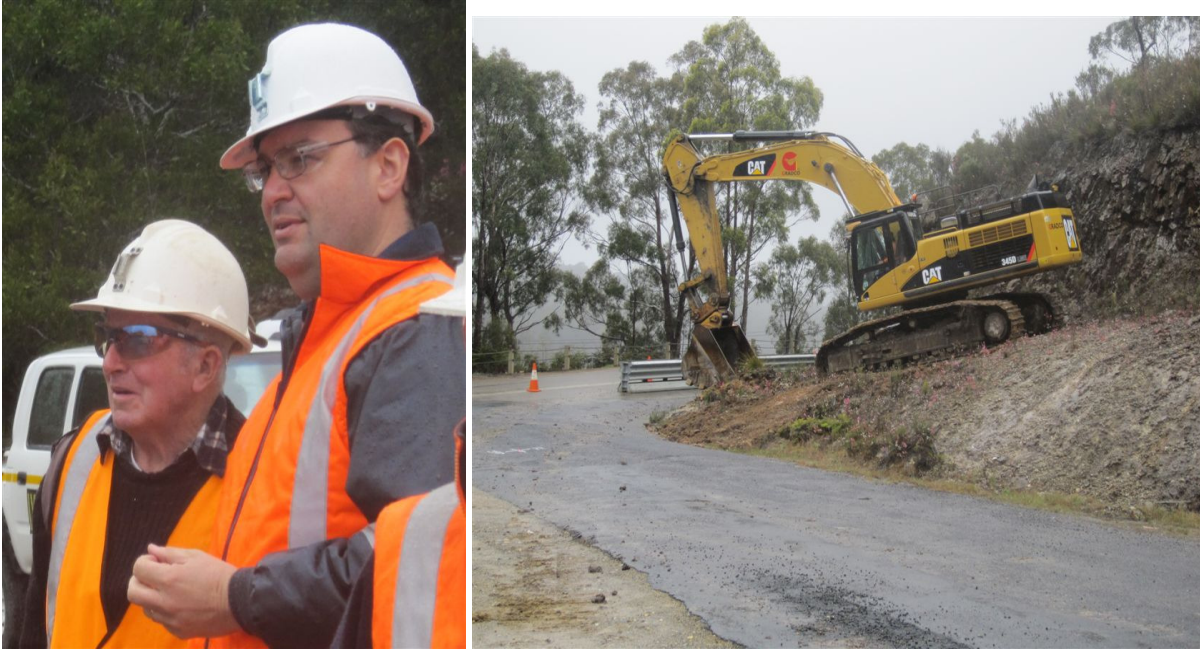
Bus operator Kerry Hay and MMG Rosebery General Manager John Lamb observe the remodelling of the Murchison Highway and Williamsford Road intersection.
