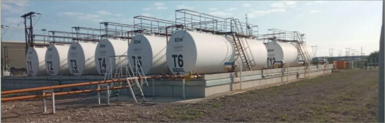
Figure 13-14 Fuel farm – Boseto processing plant
