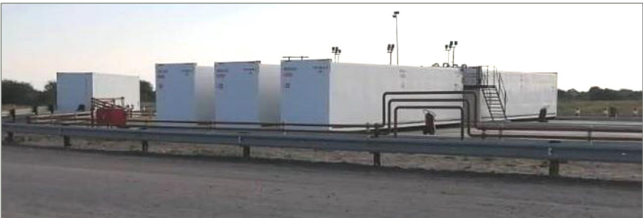
Figure 13-15 Fuel farm – Zone 5
