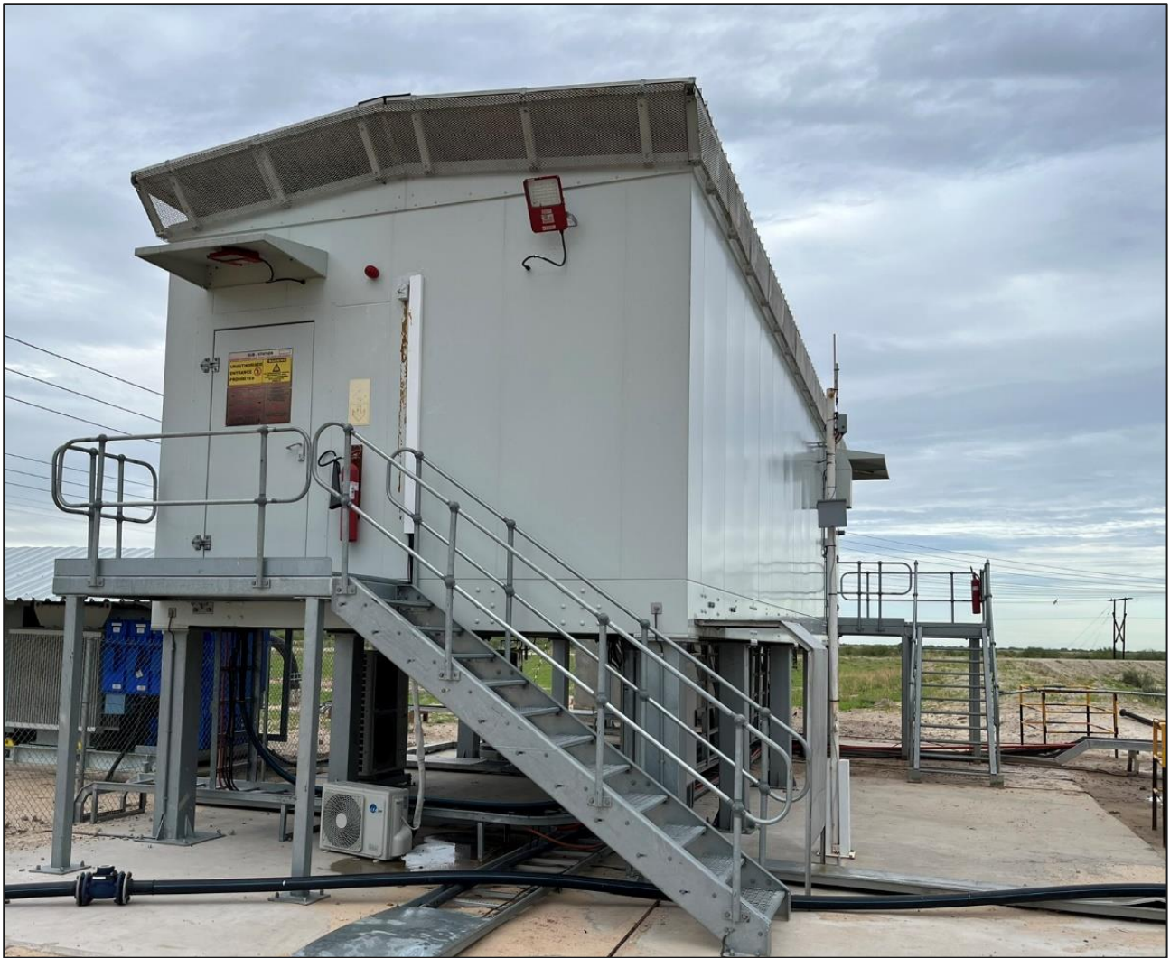
Figure 11-10 Boxcut located substation above the portal
